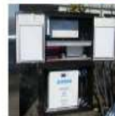
Emergency power BOX
